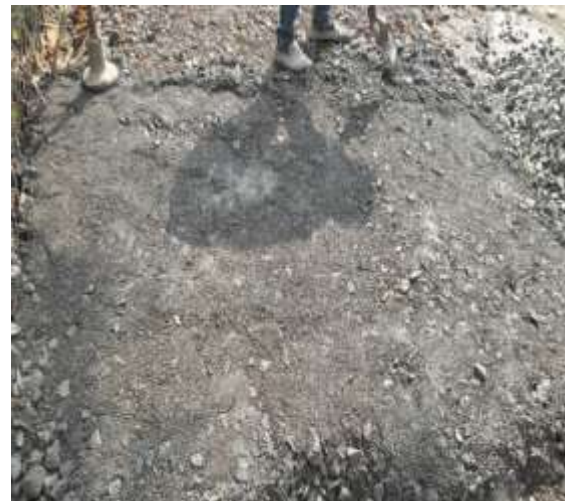
Fig. No. 6 The parking area after completion of work followed by the compaction
