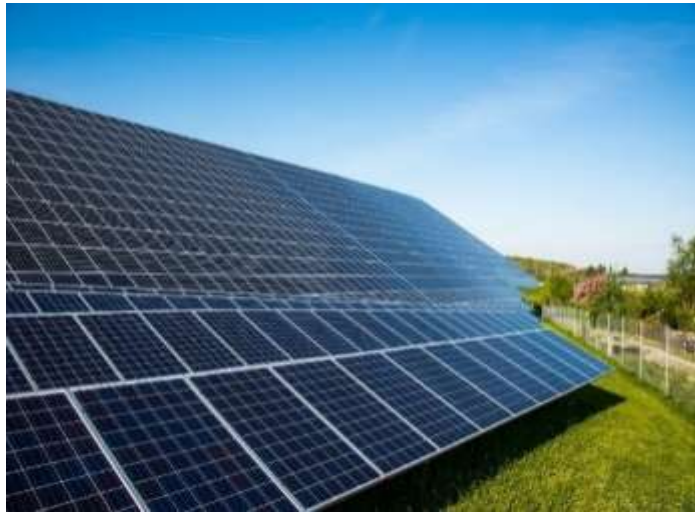
Fig.1.3 (a) Photovoltaic Panels
