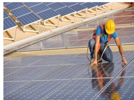
Fig-1: Solar panel.
